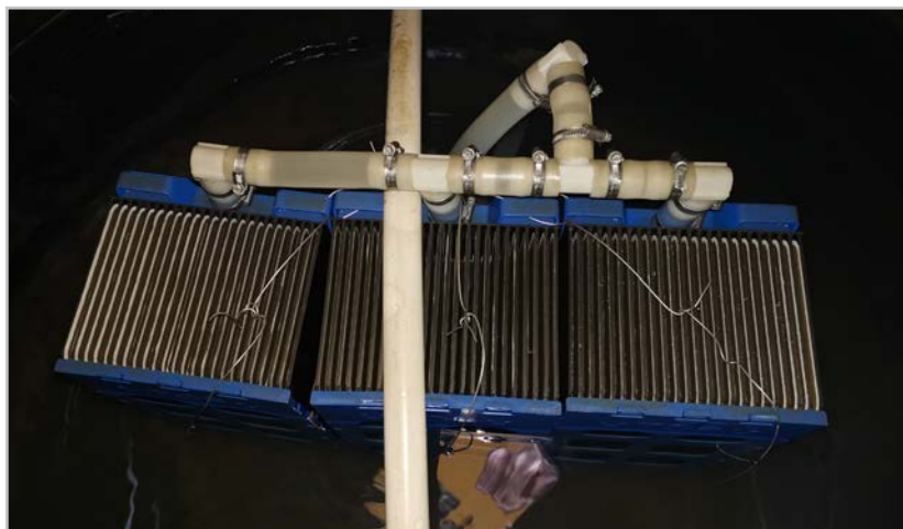
Figure 45: Three TDS-MC-MCXS2 membrane modules installed in Liberia
