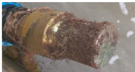
Figure 14: Clogged strainer due to lacking maintenance
