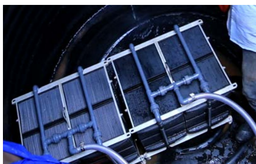
Figure 26: Aqua Cube modules in the membrane tank
