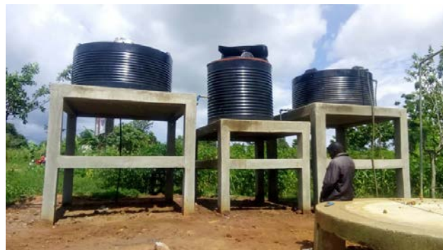
Figure 28: Fundaments of a three tank set-up
