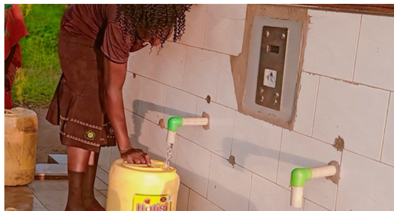
Figure 38: Automatic water vending machine (Water ATM)
