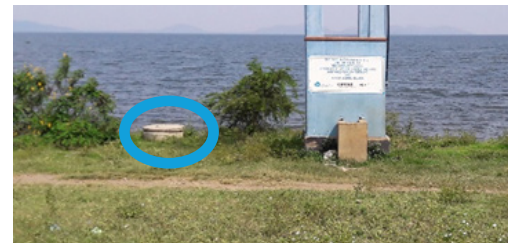
Figure 17: Picture of the pump house and the infiltration well (encircled)
