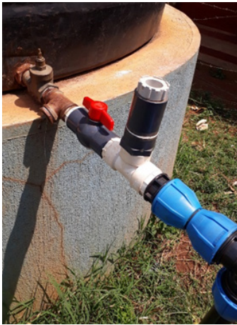
Figure 48: T-chlorinator installed after the clean water storage tank
