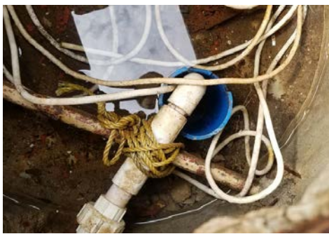
Figure 41: Groundwater well with plastic coat (blue)
