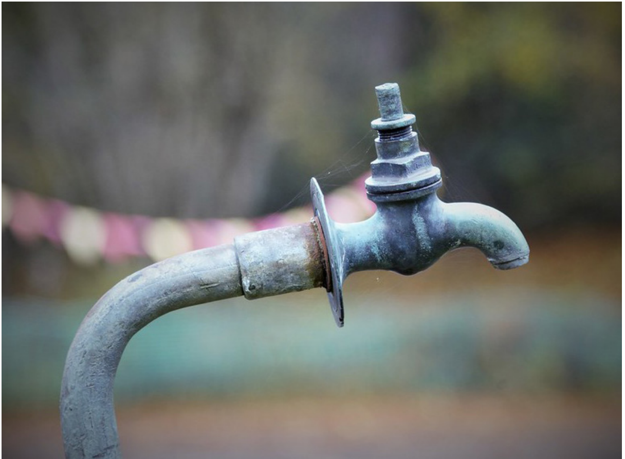
Figure 53: Non-functional water tap (© Jason Allardyce)
