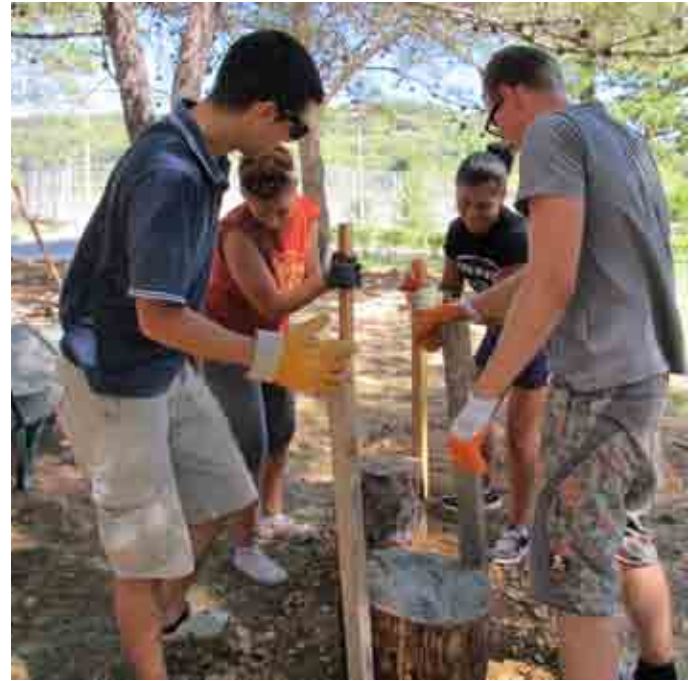
FIGURE 4. The building process is collaborative and uses ingenuity such as the home made tampers to compact the gravel.
