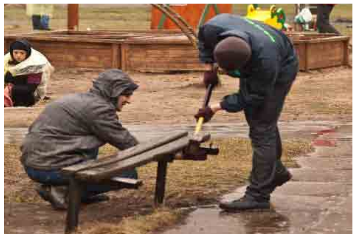
FIGURE 10. 63 S.Eizensteina street in Riga - revitalization and landscaping work labiekārtošanas darbi. (Image: Niklāvs Josla, 2013)
